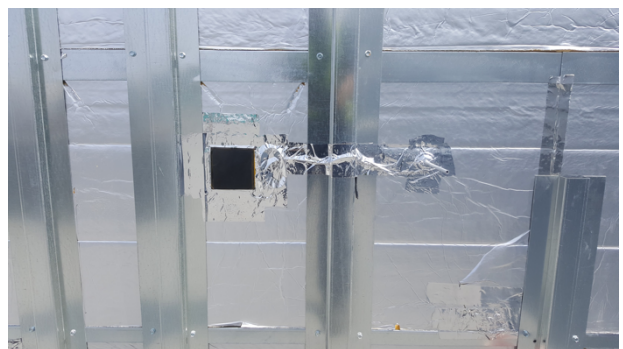
Figure 5. External Heat Flux, Temperature and Pressure Installation
