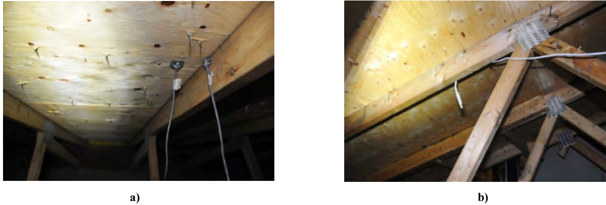
Figure 6: Field Observation in the Attic of House II: no Signs of Moisture on Building Materials and no Rusted Roofing Nails
