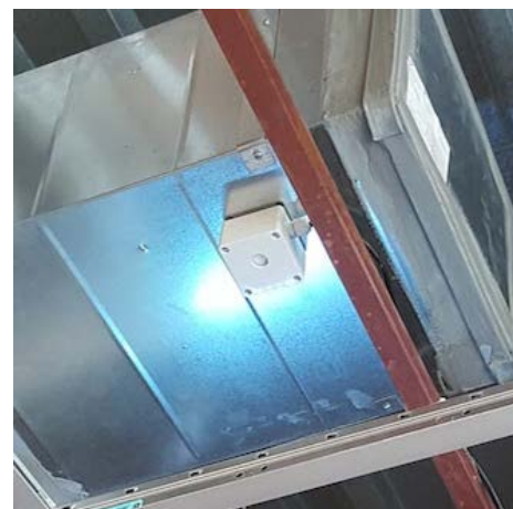
Monitoring CO 2 around ductwork
