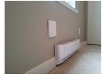
A3 installed in living space
